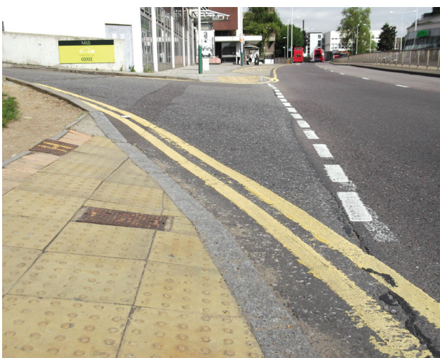
Poorly aligned tactile paving at an uncontrolled crossing, evidence of vehicle overrun small cut pieces of paving and a long crossing distance
