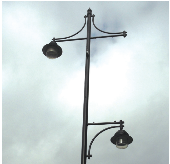
Lighting column with supplementary task lighting for a footway
