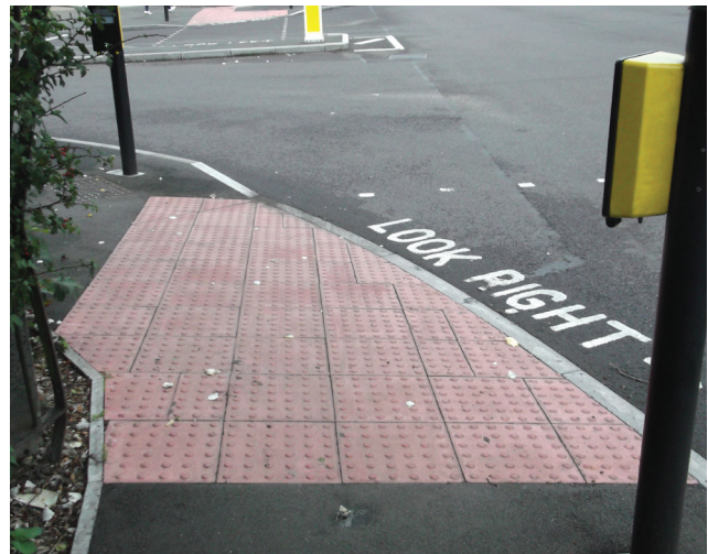
Tactile paving laid in a way that could confuse people into walking across the road at an unintended location road
