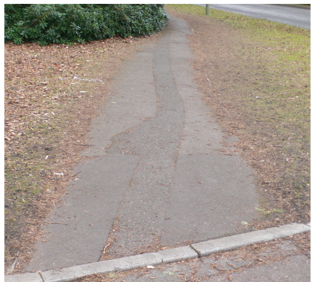
Poorly laid dropped kerbs will not be accessible to all
